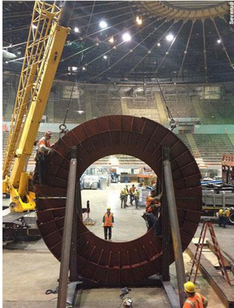
Workers prepare to raise a new steel compression ring, more than 20 ft in diameter, to the ceiling of the Forum. Severud
