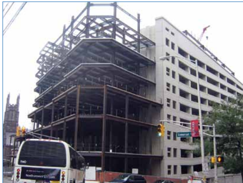
Precast Garage Supports both Lateral and Gravity forces from the Steel Structure.
