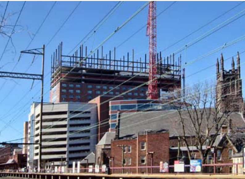
◀ The project, under construction, with train station and Amtrak wires in the foreground.
